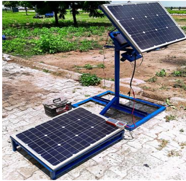
Plate 1. Assembled microcontroller based and the fixed mounted PV system
